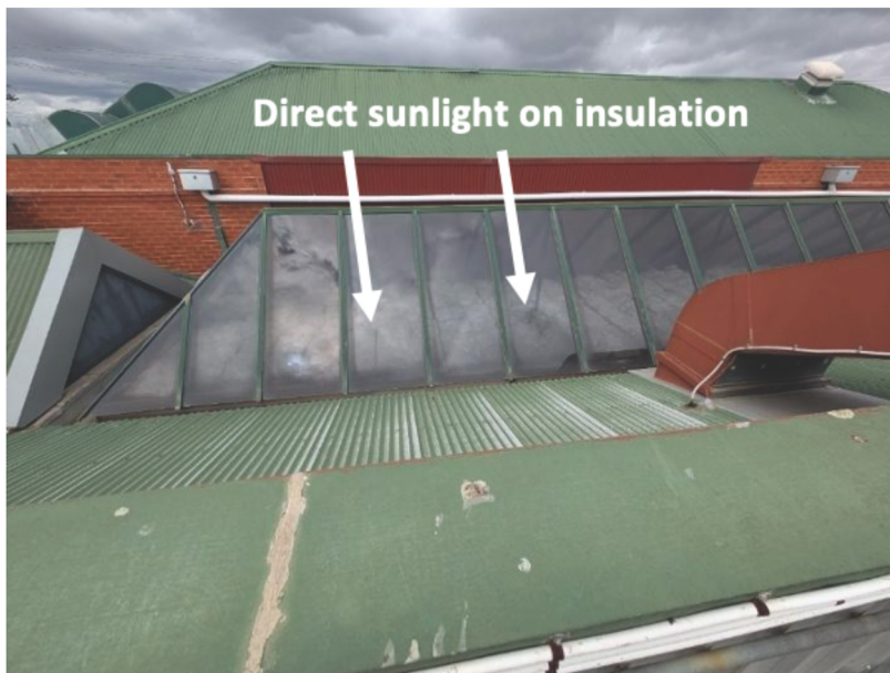
Figure 4. Legacy Roof Issues with Insulation
