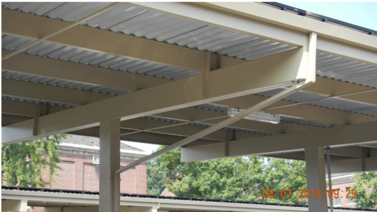
Figure 5. Corrugated roof decking allows easy mounting of panels, but blocks use of bi-facial panels. (Photo credit: Lindsay Audin)
