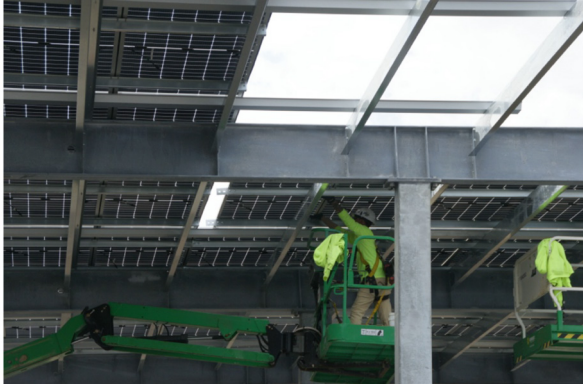
Figure 13. Panel assemblies being inserted into a metal frame racking system. (Photo credit: David. S. Goldman, used with permission)
