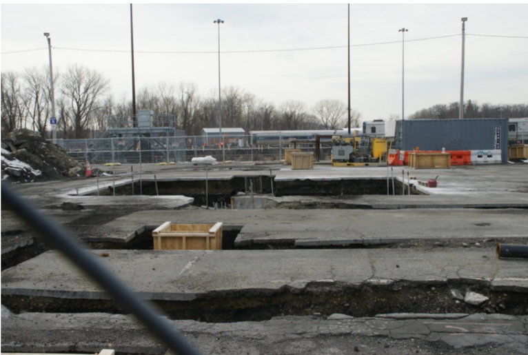
Figure 18. During construction, excavations to accommodate underground power conduits may create large craters and trenches. (Photo credit: David. S. Goldman, used with permission)
