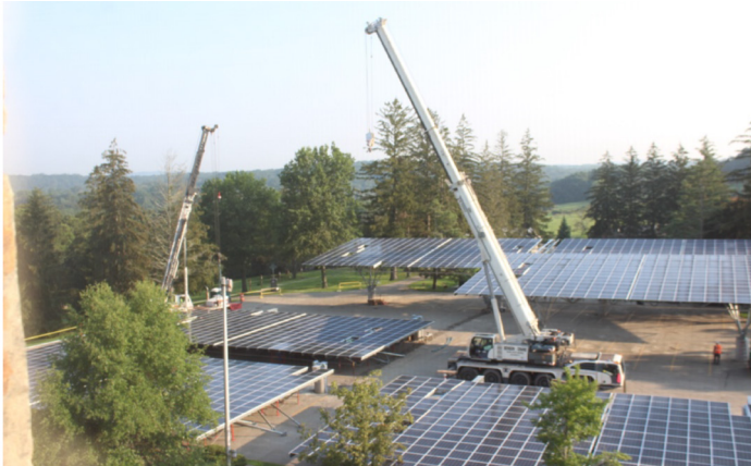
Figure 14. Another racking system involves assembling an entire canopy on the ground and lifting it into place using two large cranes. (Photo credit: Brock Gibian, used with permission)
