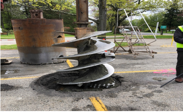
Figure 11. An auger drill on a small crawler digs holes for concrete piers. (Photo credit: Brock Gibian, used with permission)
