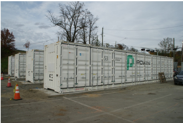
Figure 7. The Croton system includes a 3.5 MW BESS consisting of four 25-ton enclosures. (Photo credit: David S. Goldman, used with permission)
