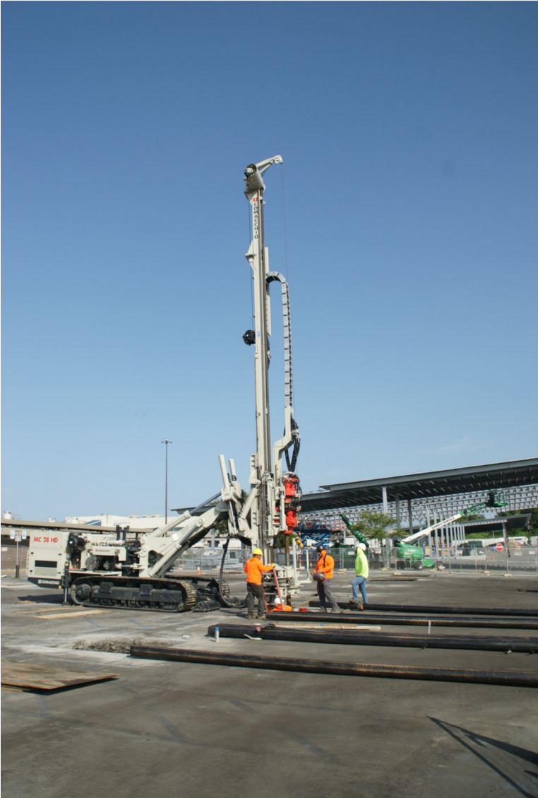
Figure 9. To dig deep holes for micropile supports, a large crawler drill is needed. (Photo credit: David. S. Goldman, used with permission)
